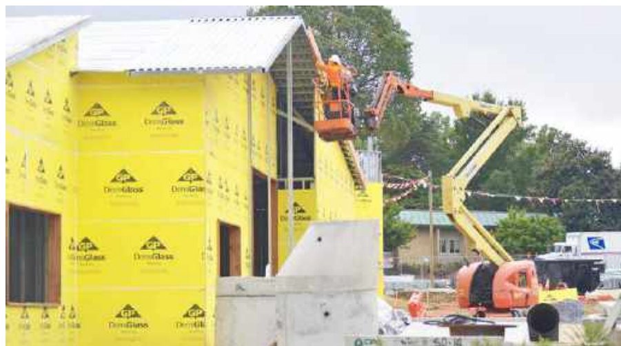
A worker adds roof framing to the coming Administration Building on Sept. 29. Photo by Leisure World News
